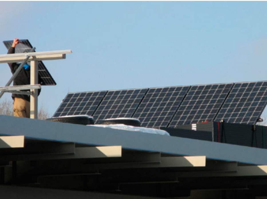
Solar panels atop the Car Rental Canopy provide a source of renewable energy for the airport.
